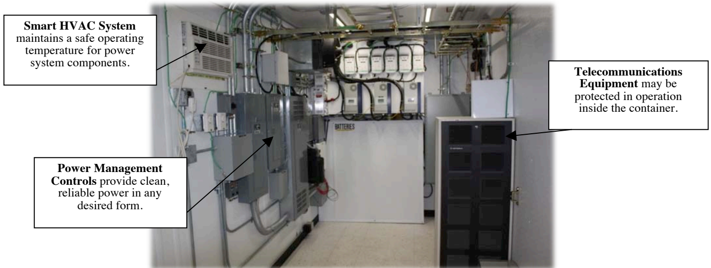
Figure 4: An example interior of a SkyStation powering a communication site. NOTE: This figure is shown for illustrative purposes only; actual installed equipment and system configuration may vary.
