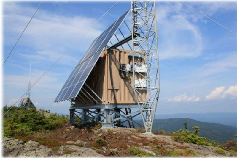
Figure 1: An example of a SkyBuilt SkyStation powering a remote communication site. NOTE: This figure is shown for illustrative purposes only; actual installed equipment and system configuration may vary.
